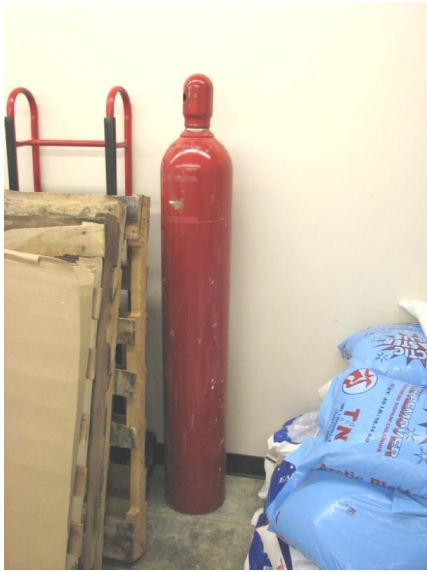
UNSAFE: Un-labeled gas cylinder that is not chained to the wall. This cylinder does have the protective valve cap in place.
