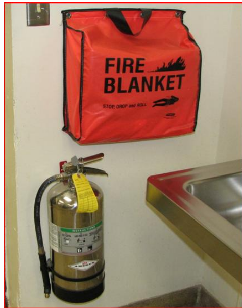
Keep fire extinguishers clear.
