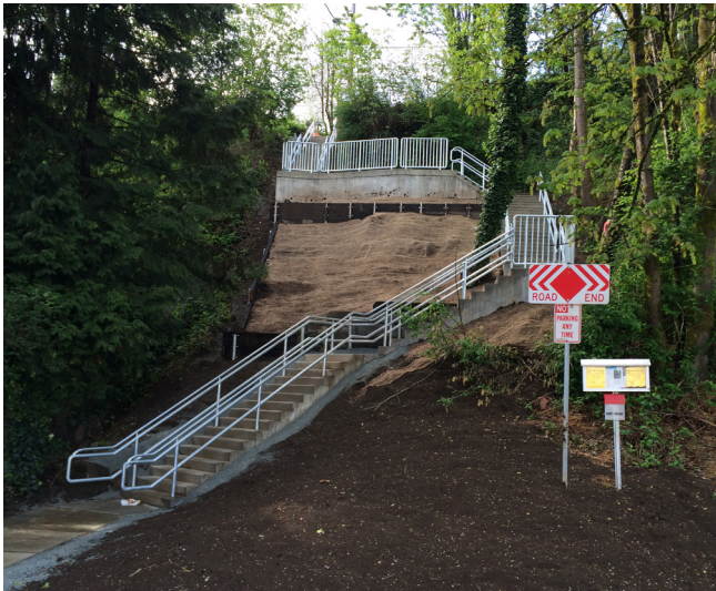
Rehabilitated stairway on 12th Ave S between S Trenton and S Concord streets built in 2016.
