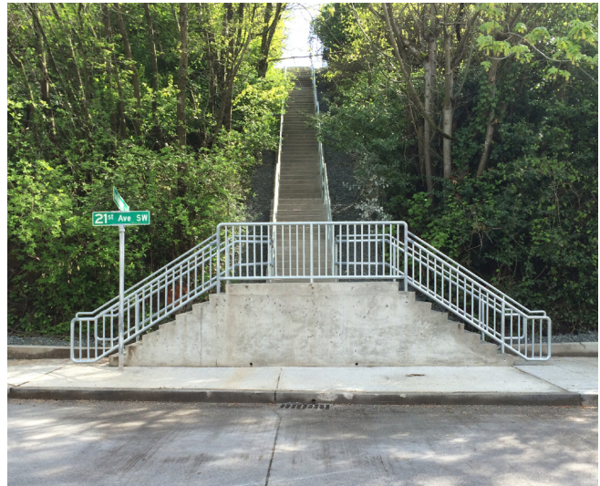
Rehabilitated stairway SW Andover St between 21st and 20th Ave SW built in 2016.
