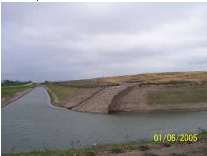
Riprap drainage way off final cover into perimeter sedimentation pond at Clay County Landfill.
