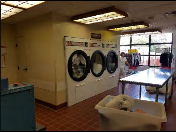
LAUNDRY BUILDING- DRYERS
