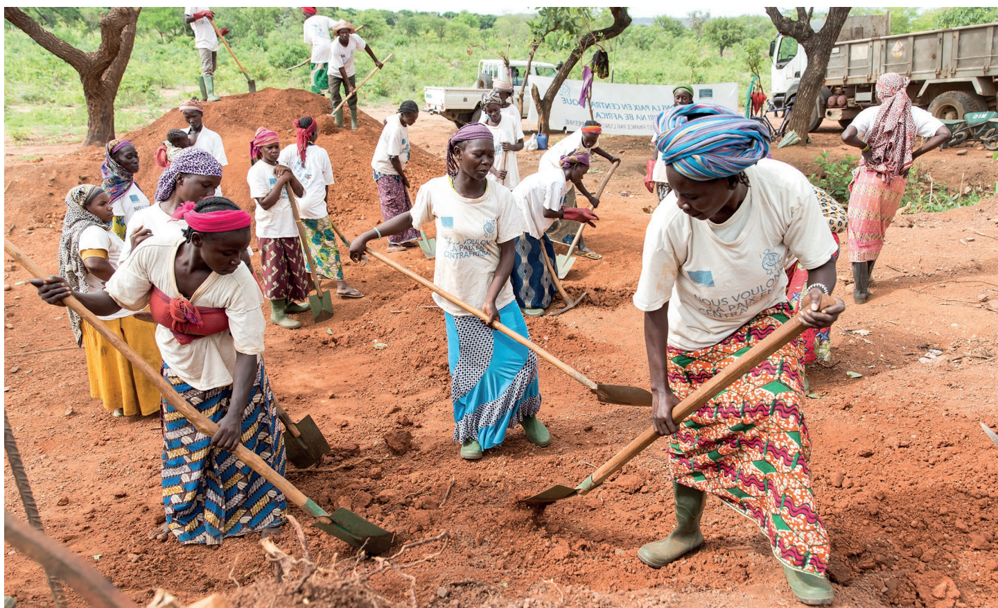
ONGOING SINCE 2014, IOM'S COMMUNITY STABILIZATION AND EARLY RECOVERY PROJECT SIRIRI, FOCUSES ON REVITALIZING LOCAL MARKETS INCLUDING THROUGH CASH-FOR-WORK ACTIVITIES; REHABILITATION OF COMMUNITY INFRASTRUCTURES (SCHOOLS, MEDICAL FACILITIES AND SOCIAL CENTRES); AND STRENGTHENING INTERCOMMUNITY DIALOGUE AND PACIFIC COHABITATION. © IOM 2017/ AMANDA NERO
