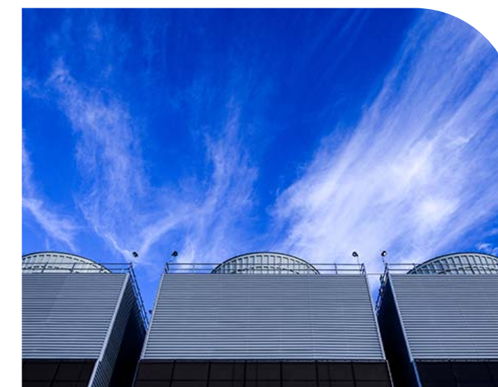
The cooling towers at our Mayes County, Oklahoma data center help keep our servers running efficiently.
