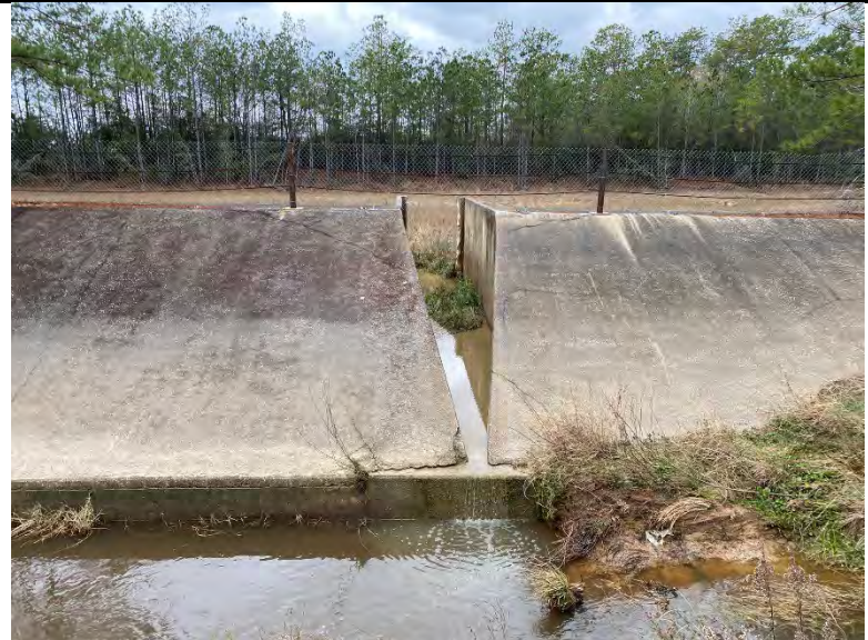
Photo IMG-2030, view of stormwater detention basin SC1 outfall into the unnamed tributary UT-1.
