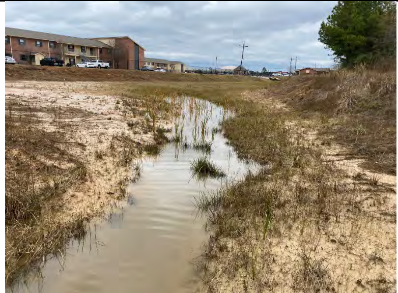
Photo IMG-2051, view of Ditch 2 where it receives stormwater flow from the offsite stormwater detention basin.
