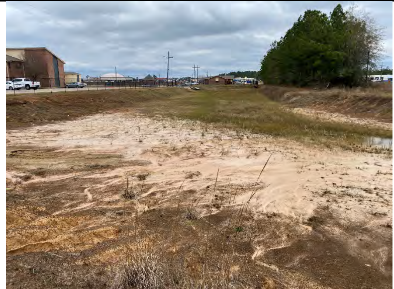
Photo IMG-2047, view of stormwater detention basin at the upper reach of Ditch 2.
