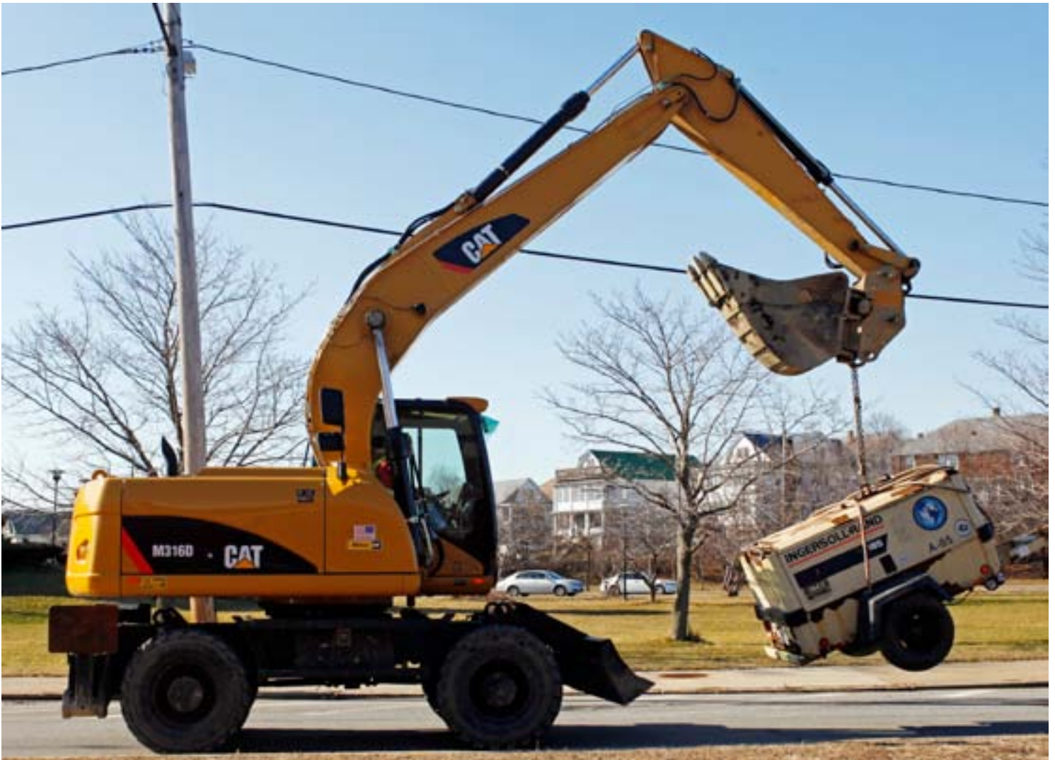
METAMORPHOSIS: A Caterpillar tractor lifts a piece of construction equipment in Somerville, Massachusetts January 27, 2010. REUTERS/BRIAN SNYDER
