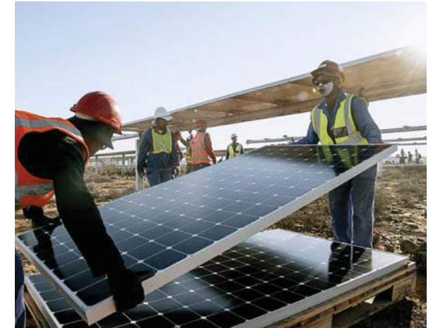
Total SunPower solar power plant, Prieska, South Africa.
