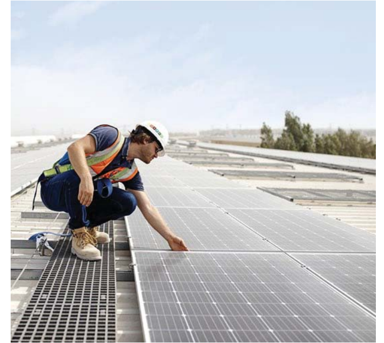
Solar panels on a roof, United Arab Emirates.
