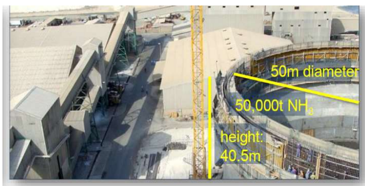
Figure SI 4.2 Ammonia storage tank in Qatar
