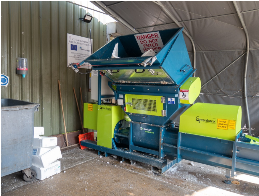
Figure 35. Photo - EPS Compressing machine in Billingsgate market
