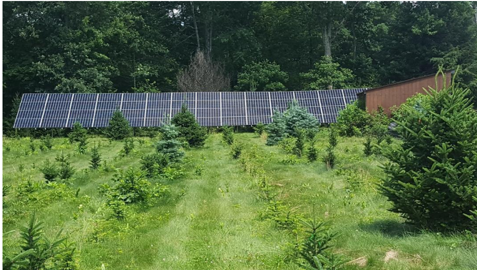
Figure 5: Ground mount solar system at Bedrock Tree Farm, Wakefield, RI. This array offsets 100% of electricity usage, with a payback period of only 3-4 years. Three different programs were used for the funding of this project: RIAgEP, REAP, and the Renewable Energy Fund.
