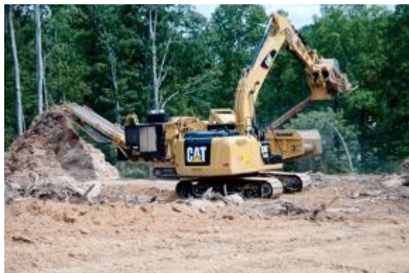
Fig. 4.12. Uranium Processing Facility site readiness construction used a mulcher/chipper to produce mulch that was used as erosion control along the haul road.
