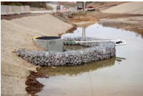
Fig. 4.11. Faircloth skimmer previously installed at Sediment Basin 1.
