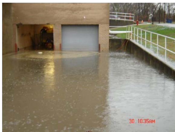
Figure 23: Westerly’s lower garage filling with overflow from the overwhelmed plant uphill on March 30 th , 2010. Eight feet of water eventually found its way to this low spot. (Westerly)
