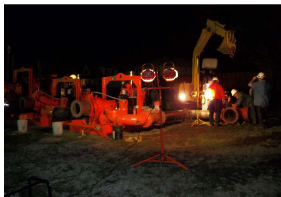
Figure 20: Bypass pumping being assembled at the Pontiac Avenue Pumping Station. (Veolia Water)
