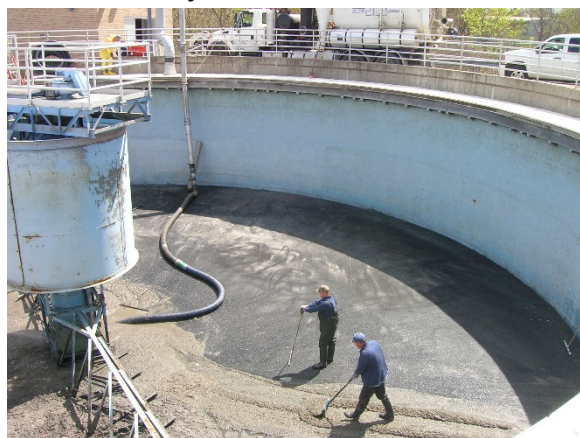
Figure 9: West Warwick staff manually pushing sludge to the center of idled primary clarifiers. From there, the sludge would be pumped away in tanker trucks. (RIDEM)
