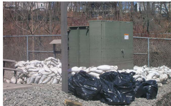
Figure 11: With flood waters long gone came remnants of frenzied attempts to sandbag critical components at the West Warwick Regional Wastewater Treatment Facility. (RIDEM)
