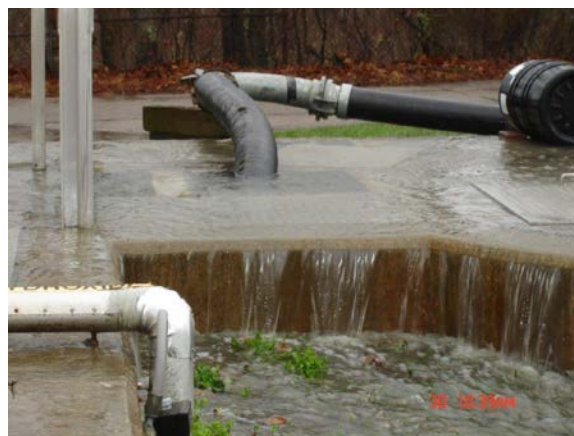
Figure 22: Heavy flows arriving at the Westerly wastewater treatment plant from townwide flooding upstream overwhelmed the plant's influent structures. Crews here have installed temporary pumping to help relieve the flow and keep it in the system. (Westerly)
