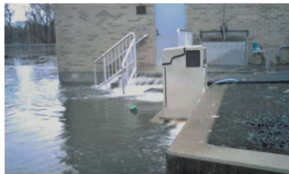
Figure 8: At higher ground, water from the flooded town makes its way into West Warwick's mostly submerged treatment facility, and out the doors of its headworks building. (West Warwick)
