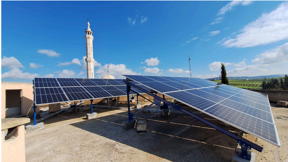
Hybrid solar photovoltaic system installed at Kafat Primary Health Centre in Hama, Syria @unops 2024
