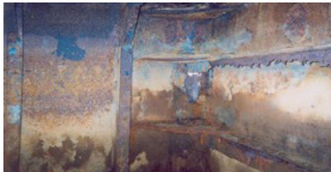
Heavy wastage and deterioration of internal structural members
