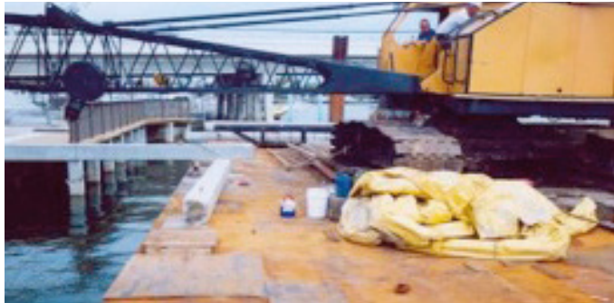
Plywood sheets cover holes in the deck. Also, the crawler crane is not secured.
