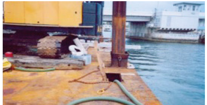
Note hole cut in deck and the portable pump & hose on deck. Barge must be regularly pumped to keep the compartment from flooding.
