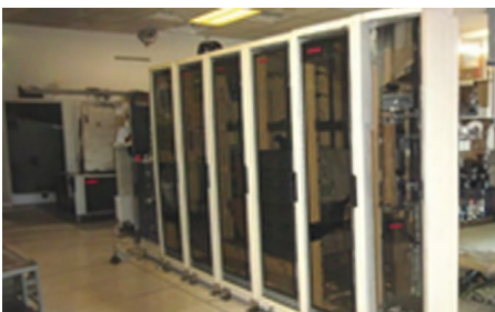
Computer server racks anchored to the floor.
