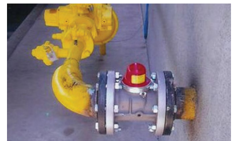
Seismic shutoff valve for natural gas line.
