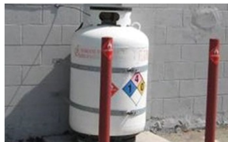
Flammable liquid tank strapped to wall.
