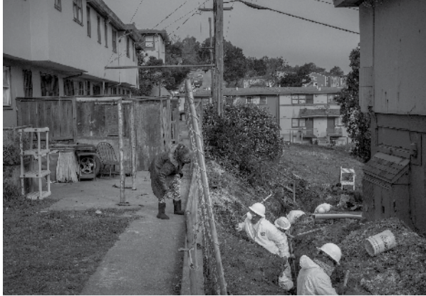
Some of the thousands of sites poisoned by the military's handling of munitions waste are in residential neighborhoods. A resident talks with construction workers in protective gear in the contaminated Hunters Point neighborhood of San Francisco. (Ashley Gilbertson/VII Photo, special to ProPublica)
