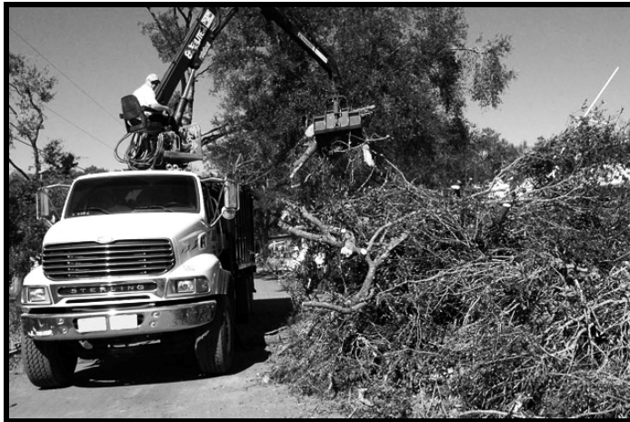
Figure 3.1 - Typical Vegetative Debris on a Public Right-of-Way
